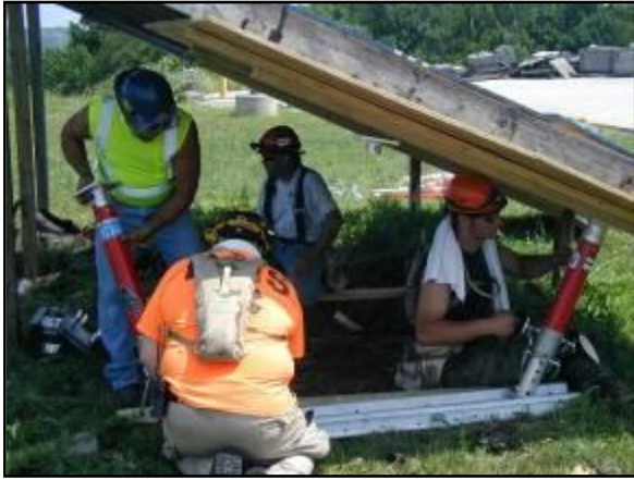
Advanced Structural Collapse team placing shores in one of the collapse scenarios.
